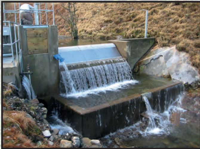
Figure 3 - Typical run-of-river intake weir. Screens (centre) allow water to drop into a settling tank (left) where it enters the pipe (buried on left bank). The plunge pool allows fish to navigate the structure unharmed.
